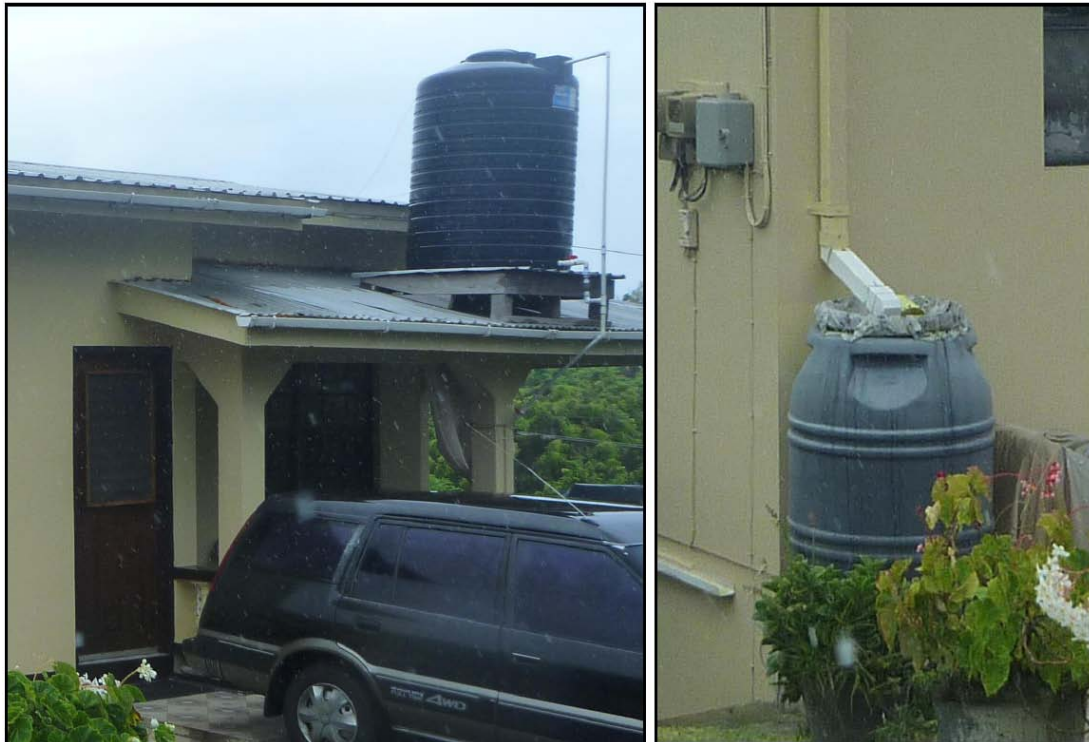
Figure 4.12. Left: Example of an elevated 500 gallon (1,890 L) black polyethylene storage tank plumbed into the home. Right: Example of a rain barrel not plumbed into the home.
