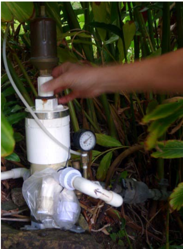
Figure 4.11. Pressure meter installed on incoming water line by a resident. This person reported diurnal pressure fluctuations between 0 psi (atmospheric pressure) and over 100 psi.
