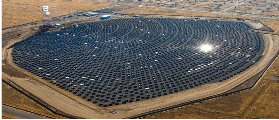
Figure 40 Bright source installation at Chevron, Coalinga
