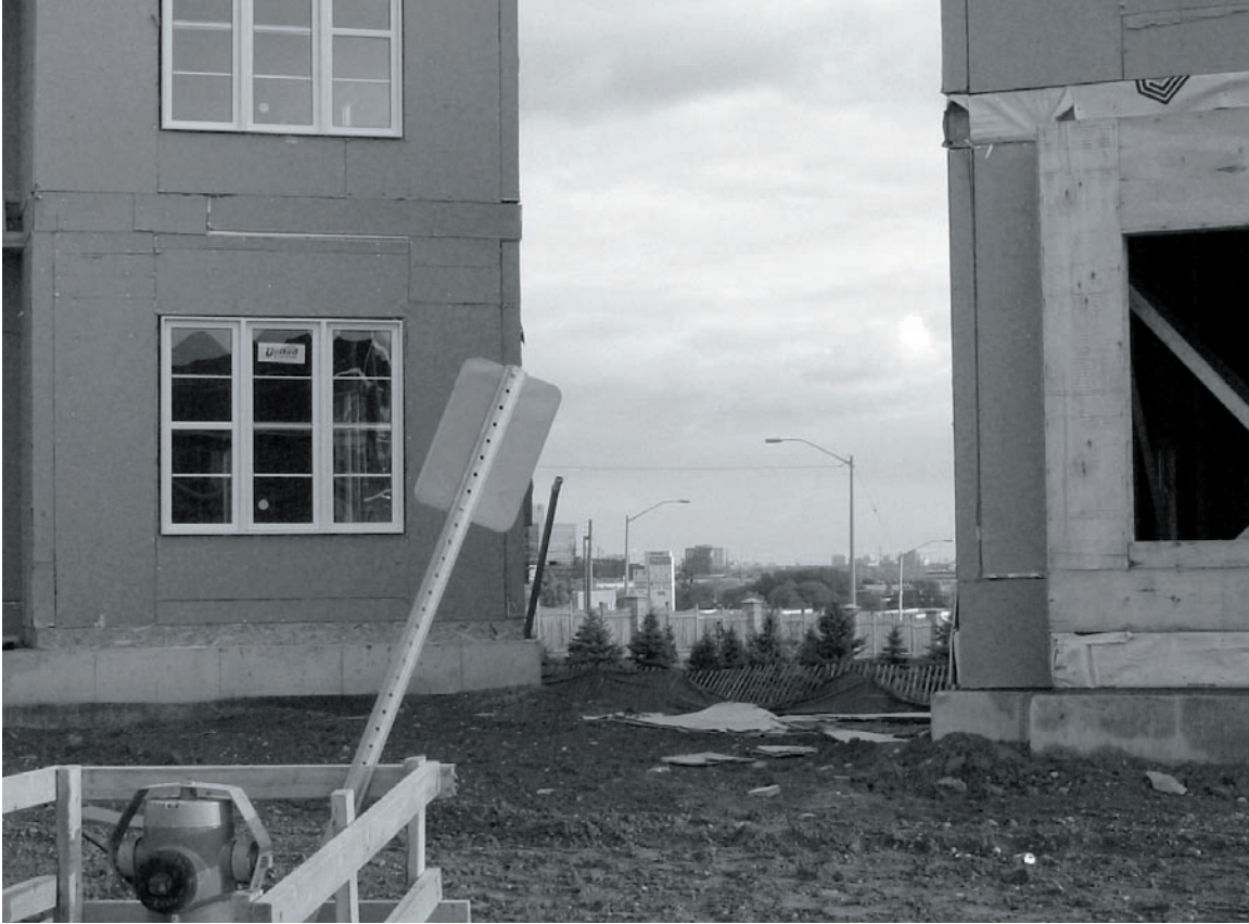
Figure 2.62 Between two unfinished homes The neighbourhood of Bayview Hills segregates itself from the social and public realm of Richmond Hill.
