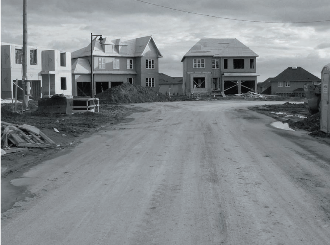
Figure 2.48 View Down unfinished road of Senator Construction Site Houses at different stages of completion reveal the developers factory-like assembly-line construction.
