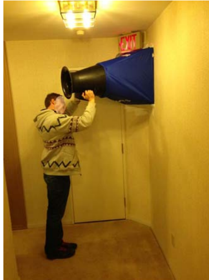
Figure 7-15: A measurement of MAU airflow supplied to a corridor being made using a balometer
