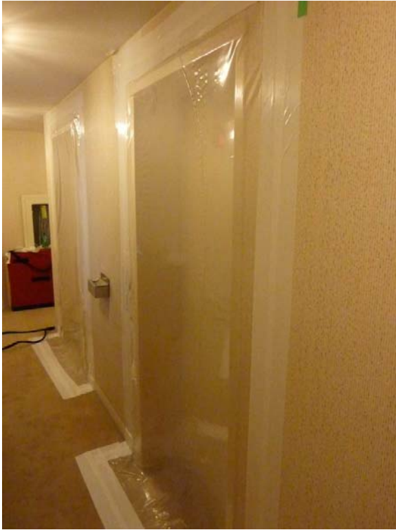
Figure 7-17: Typical sealing of elevator doors for corridor airtightness testing using polyethylene sheet and PVC tape
