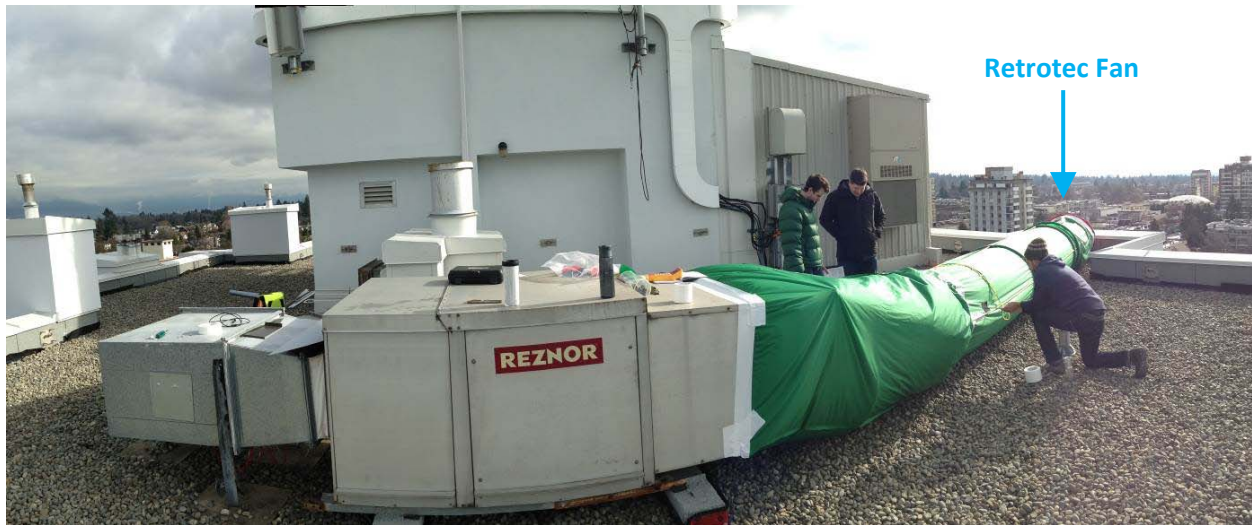
Figure 7-14: MAU testing apparatus with green flex-duct to attach Retrotec fan to the MAU intake
