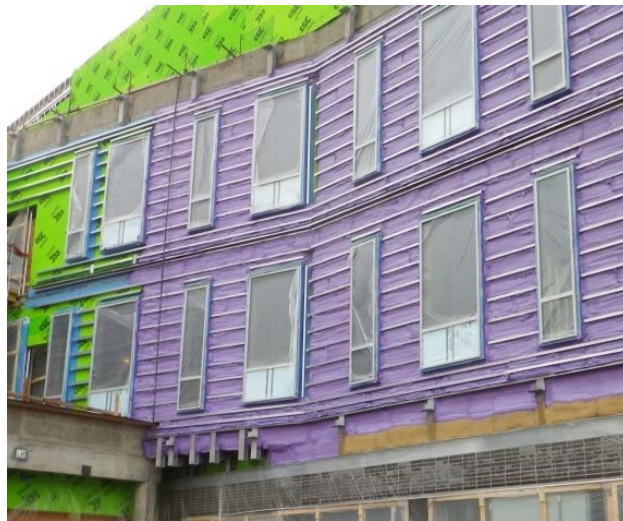
Figure 4-6: Closed cell spray foam insulation applied to exterior sheathing to provide air barrier with flexible membrane use at transitions and movement joints. (Photo courtesy of RDH.)
