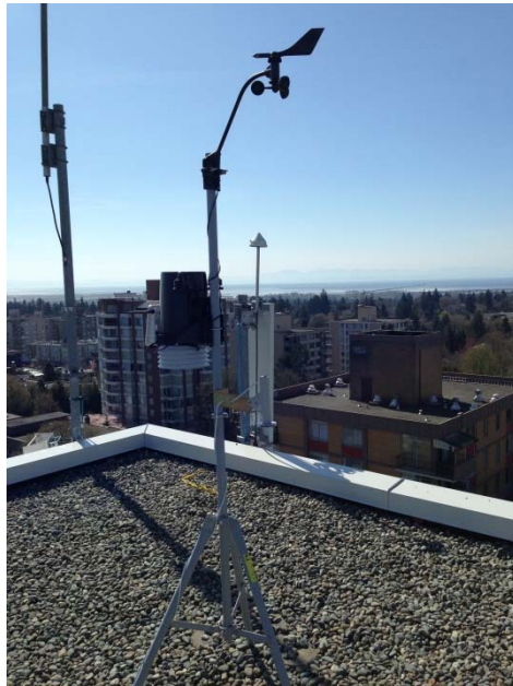
Figure 7-29: Weather station installed on roof of the case study building
