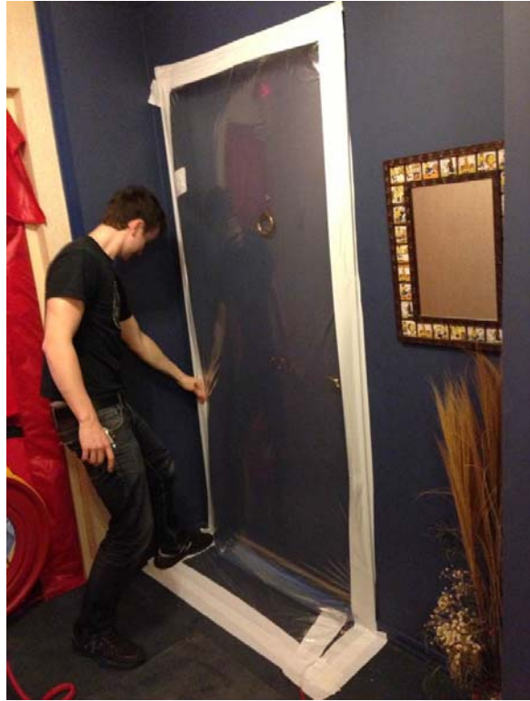
Figure 7-18: Typical sealing of suite entrance door during corridor airtightness testing using polyethylene sheet and PVC tape
