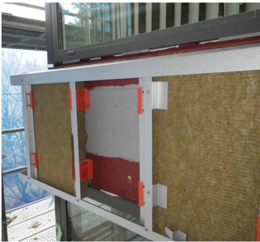
Figure 7-5: New wall assembly under construction at the case study building showing localized sealing with liquid applied membrane (red) at window head and sill, exterior mineral wool insulation, and fiberglass low conductivity clips (Photo courtesy of RDH)
