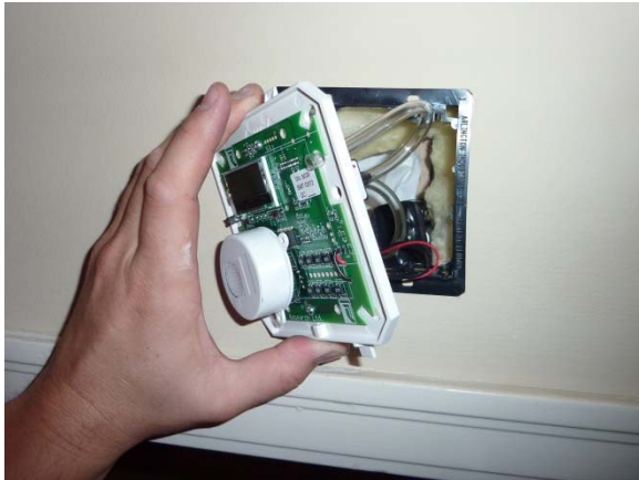
Figure 7-23: Typical SMT-A3 unit being installed in a wall above a suite entrance door
