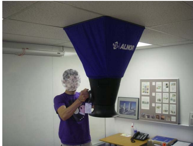
Figure 6-7: Typical Unpowered Flow Hood apparatus
