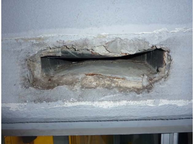
Figure 7-7: Photo of outlet of in-slab exhaust duct at the case study building showing collapsed shape of the duct.
