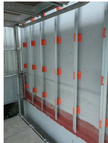
Figure 7-6: New wall assembly while under construction showing localized sealing at concrete slab cold joints, and cladding support system prior to installation of mineral wool insulation (Photo courtesy of RDH)
