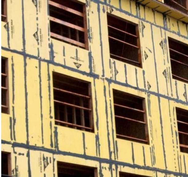
Figure 4-2: Exterior gypsum sheathing sealed to provide the air barrier. (Photo courtesy of RDH.)
