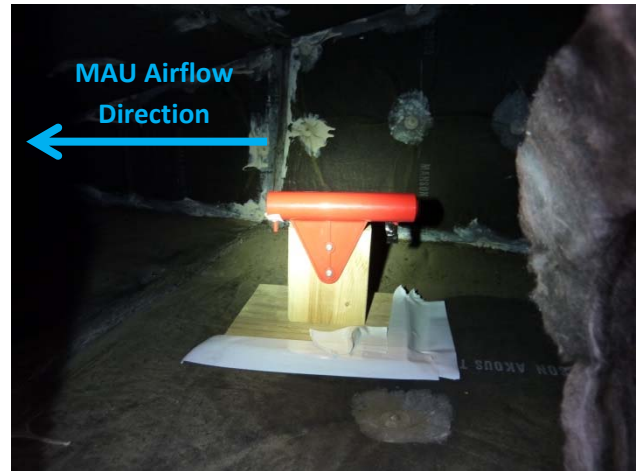
Figure C-4: Photo showing cylindrical type airflow shield containing a CATS located in the MAU duct on the roof downstream of the mega sources
