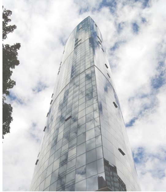
Figure 4-7: Building where curtain wall system provides the air barrier. (Photo courtesy of RDH.)
