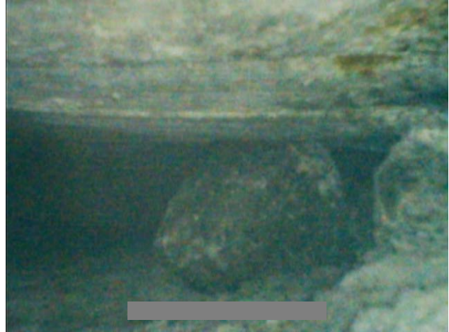
Figure 7-8: Photo of interior of a duct at the case study building showing large pieces of debris within the duct.
