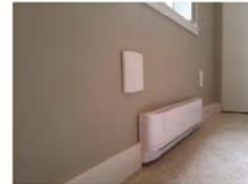
A3 installed in living space
