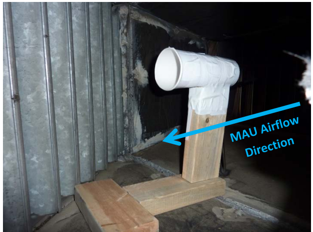
Figure C-3: Photo showing cylindrical type airflow shield containing mega sources located in the MAU duct on the roof
