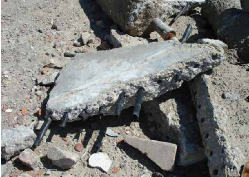
Fig. 3.13: Close up of a broken concrete floor slab with an embedded waterheating system.
