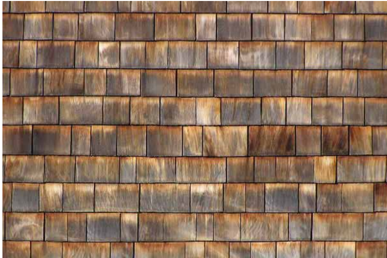
Fig. 10.20 - Cedar cladding changing colour as it weathers
