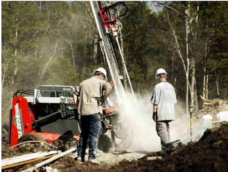
Fig. 2.9 - Geothermal technology requires installers to thread pipe into a hole a few inches wide and over 100 feet deep. This goes against Aboriginal peoples cultural beliefs, which view the earth as a living entity and mother. As such care is generally given to minimize damage and scaring of the land.
