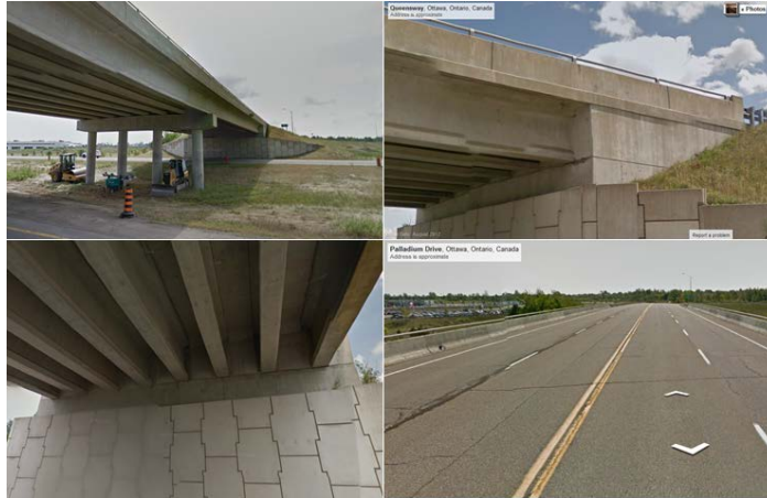
Figure 3.6: Views for PC Girders and Road Deck of the bridge (taken from Google Maps)
