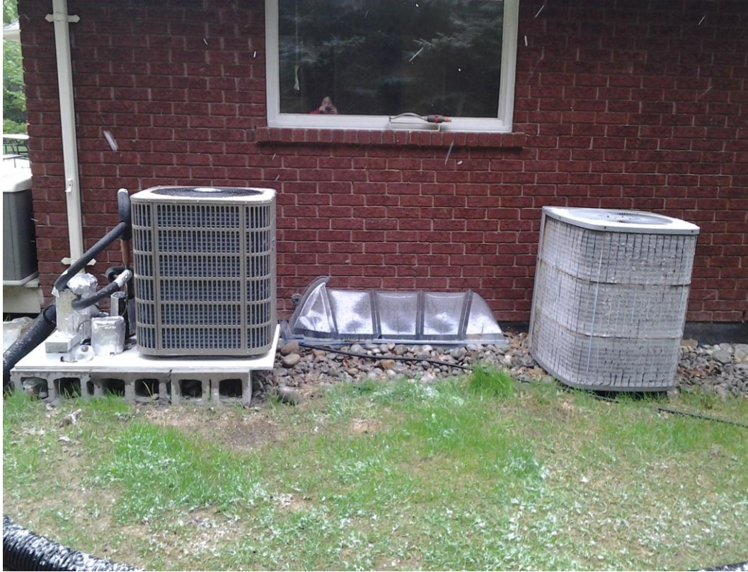
Photo 1 - High efficiency heat pump (left). Commercial Carrier heat pump (right)
