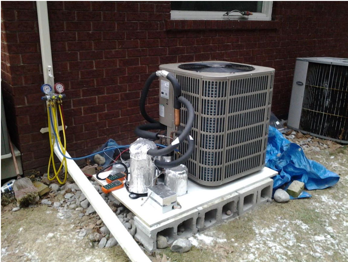
Photo 3 - Finished Unit During Charging
