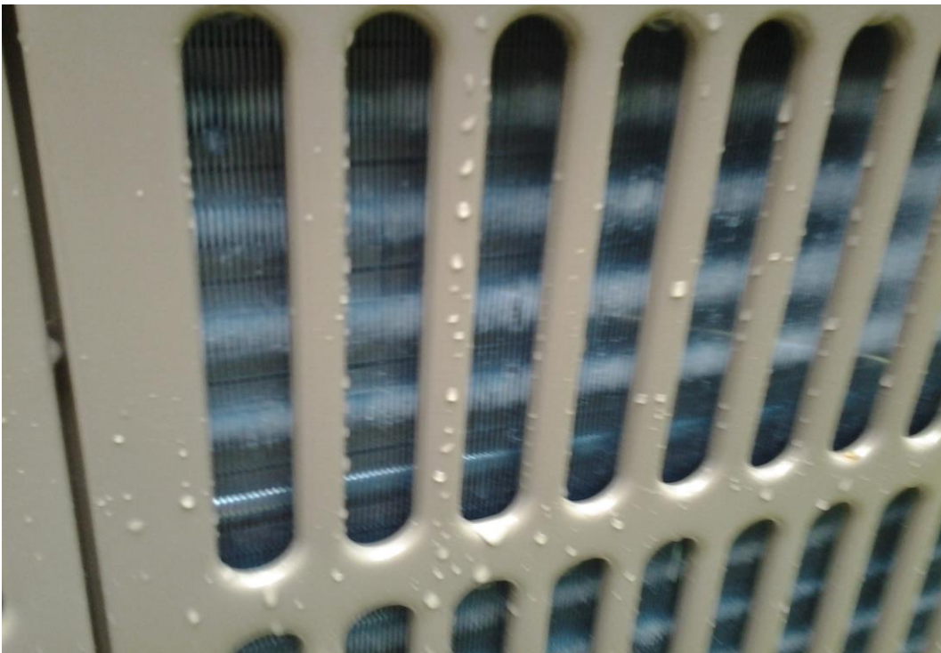
Photo 2 - High efficiency heat pump, frost accumulation at end of test.
