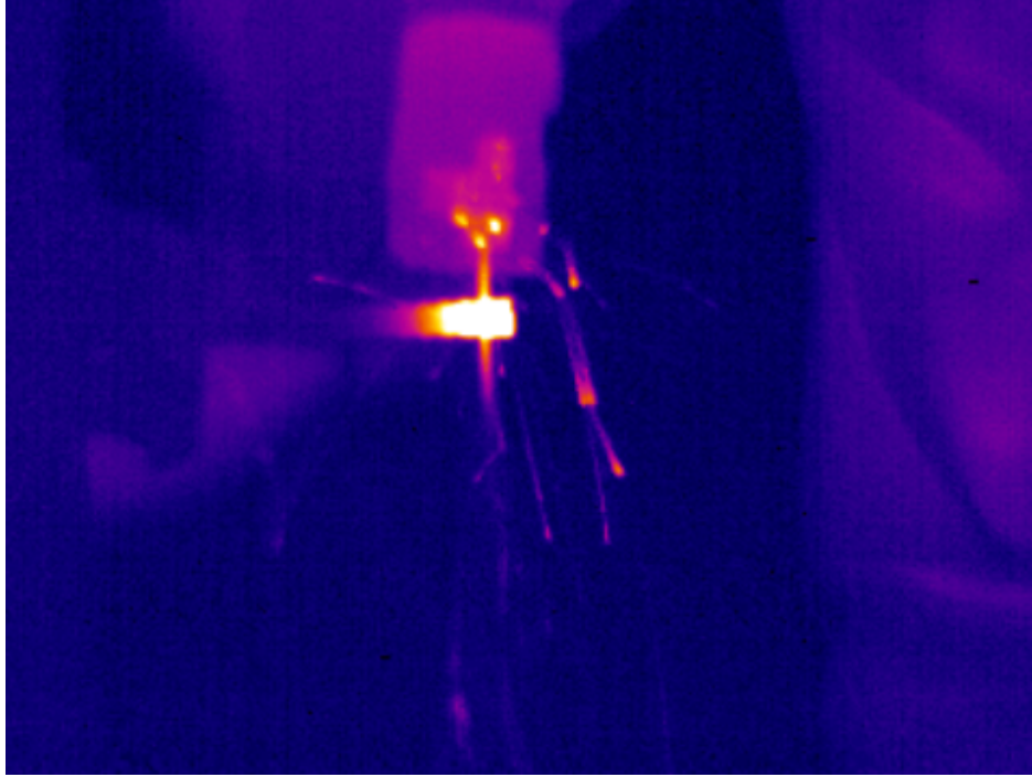
Figure 4.15: IR Footage showing hot particles leaving the rebar prior to separation during the cut
