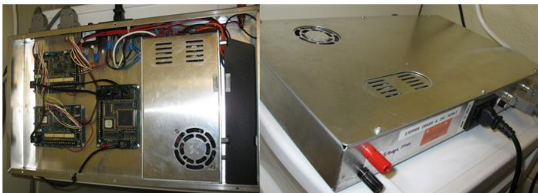
Figure.3.29 Electrical components enclosed in a case.
