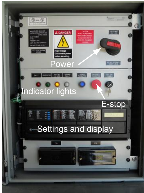
Figure 3.15: Front panel of G30 controller. All settings and control may be accessed remotely, so this is only used for trouble-shooting and powering on and off the controller.
