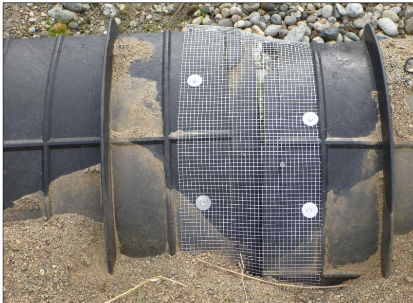
Figure III-2. ACO polymer fencing repair. Notice at the top of the fence, the section snapped off its joining part. Sand levels are also low in some areas (as shown), where they should be creating an earthen ramp over the fence for any small wildlife caught on the road side.
