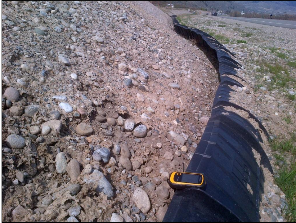
Figure III-3. Amphibian fence proximity to slope with minimal backfill; poor planning for vegetation maintenance and easily jumped by small wildlife.
