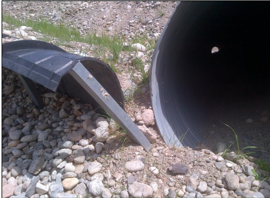
Figure III-1. Separation of ACO polymer amphibian fencing from culvert (later repaired with wire mesh overlay), Highway 97 Osoyoos passing lanes.
