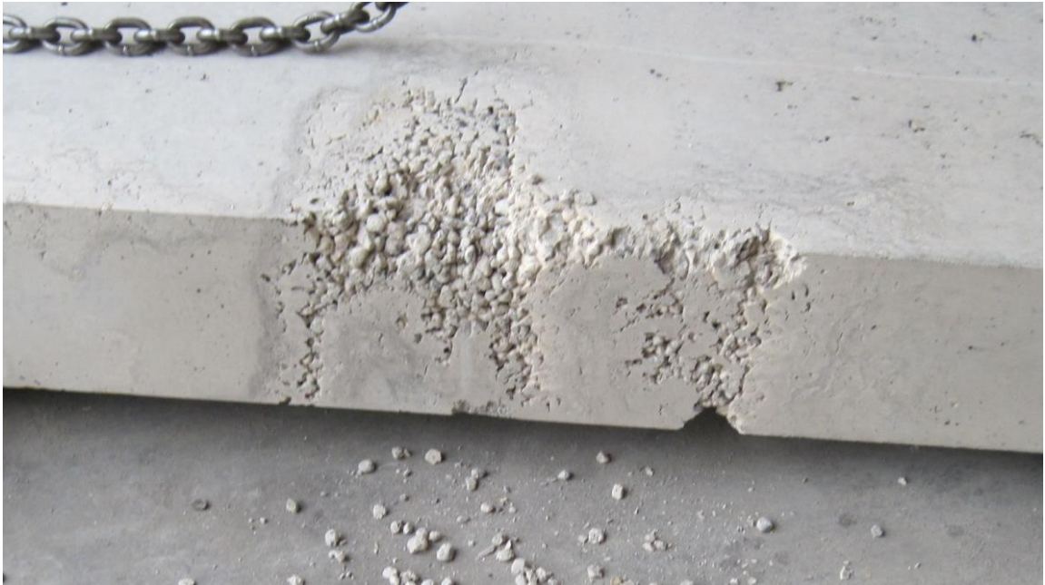
Figure 3.8: Segregation present on control wall specimens
