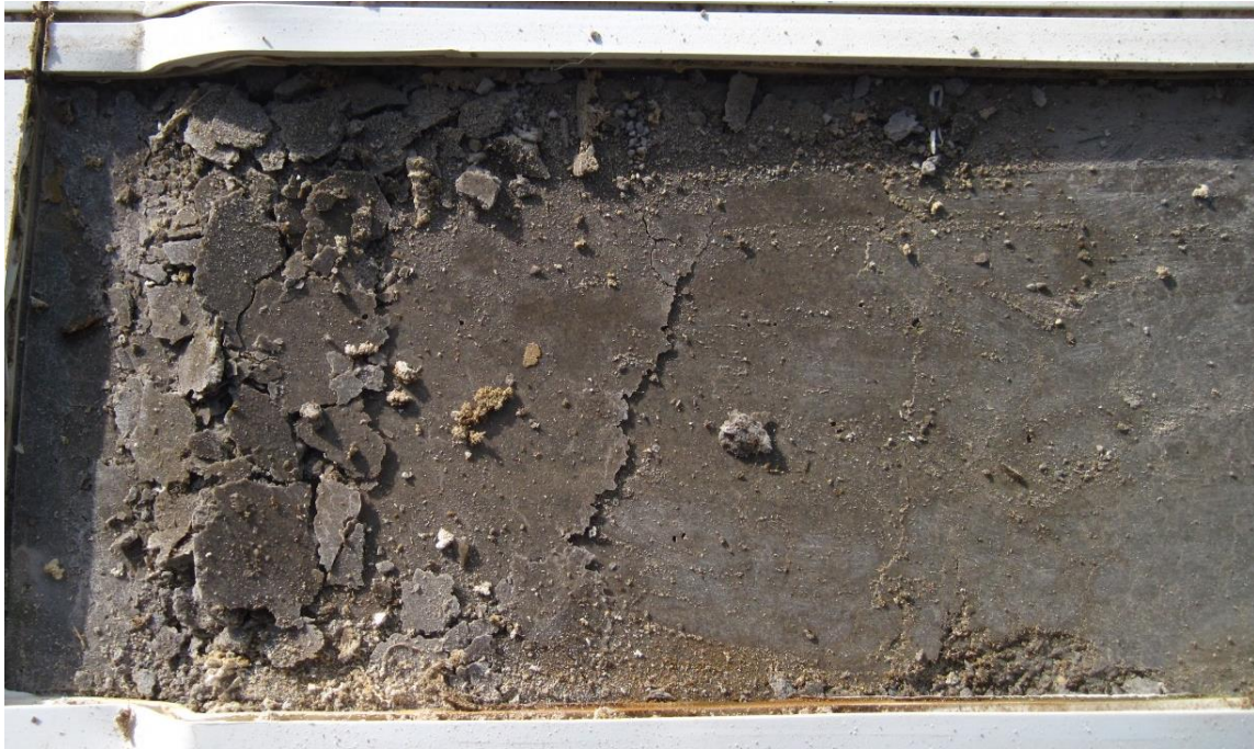
Figure 4.33: Failure location and smooth surface of hollow panel formed concrete.
