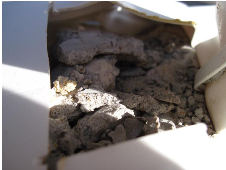
Figure 4.31: Pulverized concrete under bubbled location.
