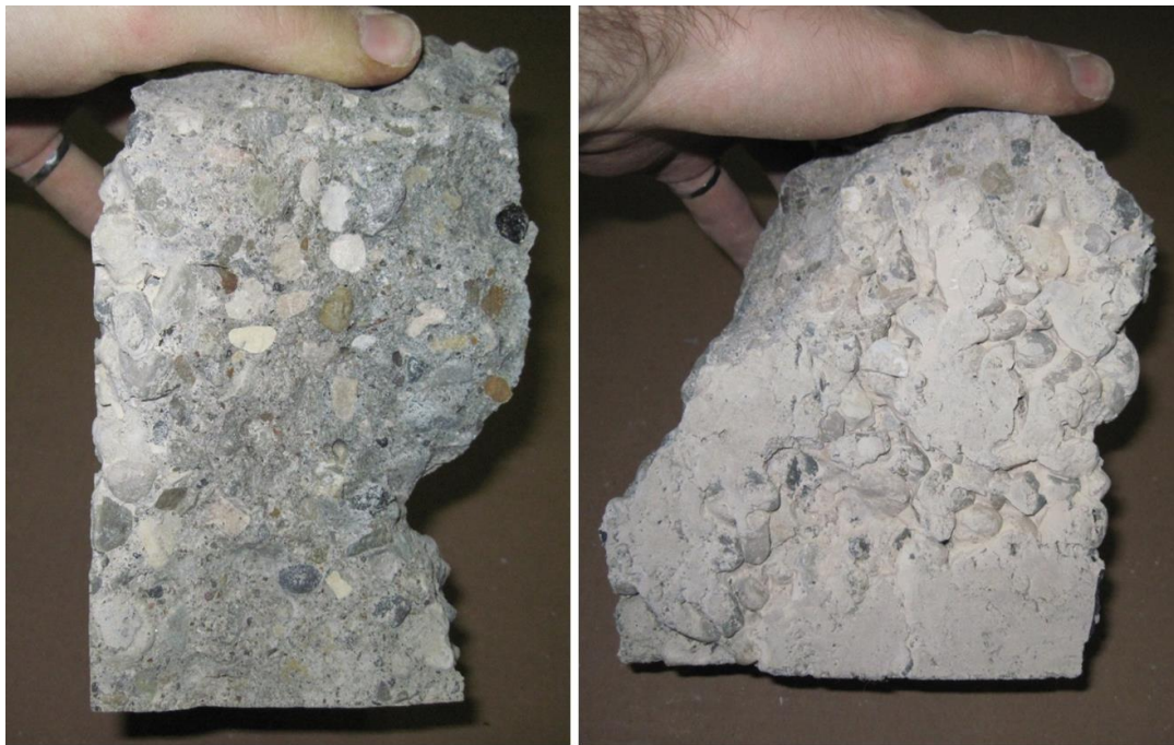
Figure 4.3: Example of surface damage observed on C-8-15, with solid concrete underneath.
