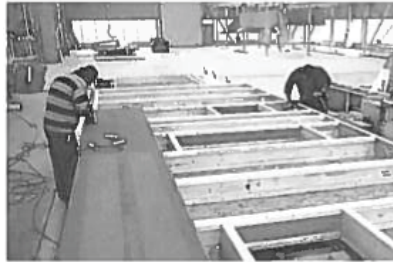
Production plant for large-format wall elements: fabrication table
