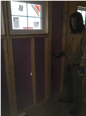
Fig. A.2.4.a. Plumbing Challenge Our plumber, Lambert, pointing to a point load he wanted to drill a hole through for a plumbing vent. We did it differently.
