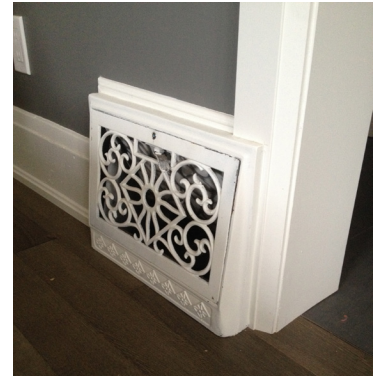
Fig. 3.4.1.3.f. Mechanical Grilles Re-used as counterpoint to the new modern elements, a consistent motif across the project.
