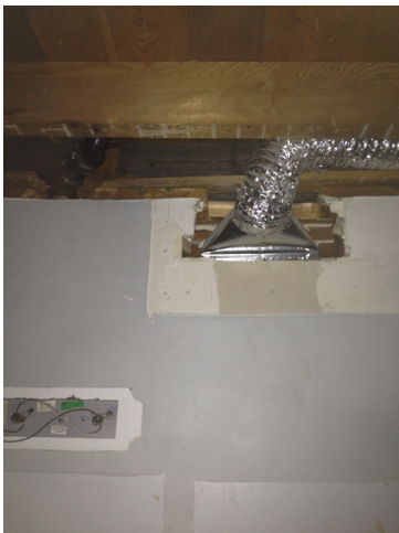
Fig. A.2.4.b. HVAC Challenge Terry, our tinbasher [HVAC installer] needed the ceiling joist notched out further to avoid a bulkhead. We decided on a bulkhead.
