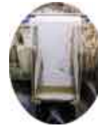
fig 3.55 outfall gates, halifax municipal treatment plant
