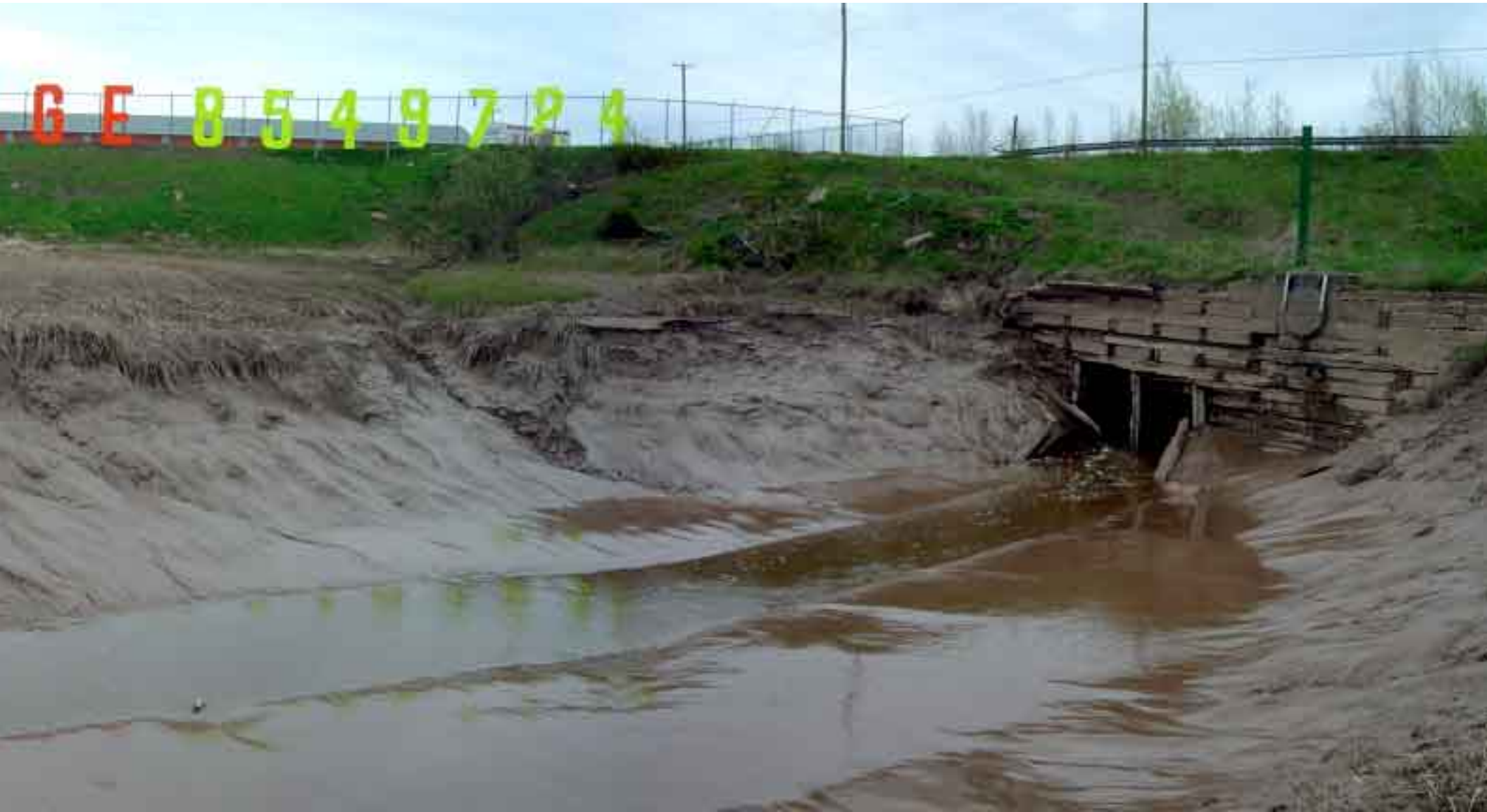
fig. 3.36 site photo. existing condition, jonathan creek flow exiting culverts under main street
