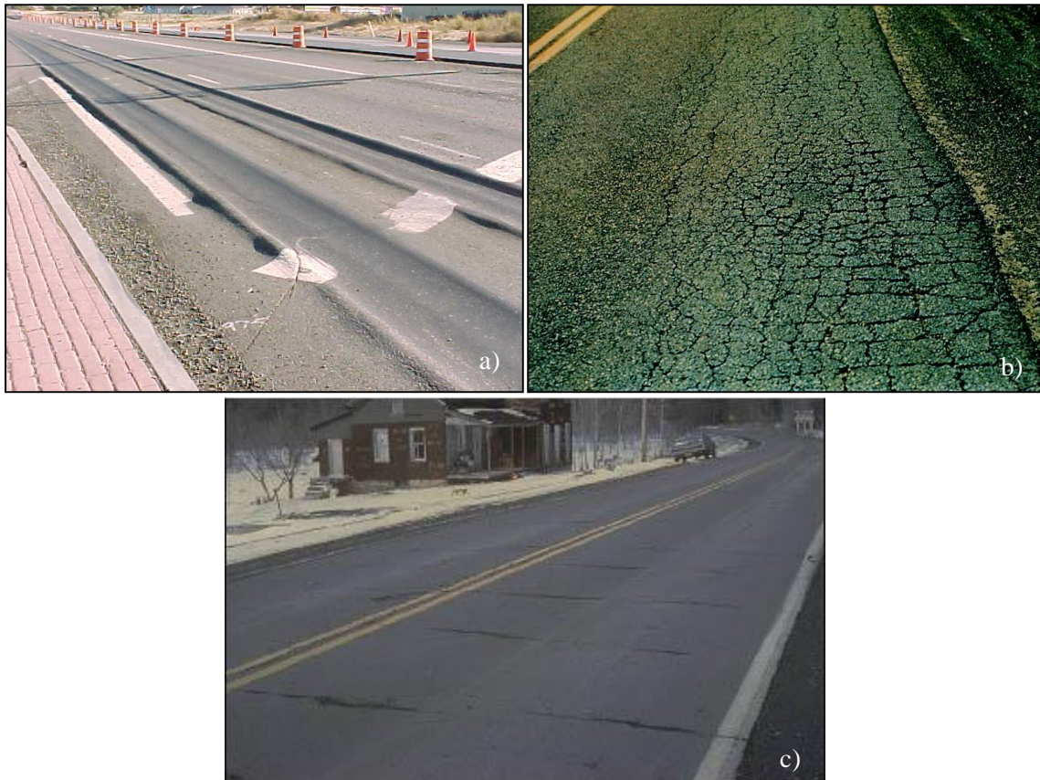
Figure 2-8 Pavement Distresses: a) Rutting (Pavement Interactive, 2008), b) Fatigue Cracking (Pavement Interactive, 2009), c) Thermal Cracking (FHWA, 2011)
