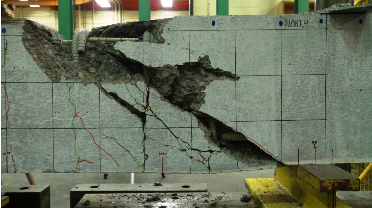
Figure E.184: BM25-150 Close-up Photo of Failure with Spalled Concrete Removed with Stirrups 11, 12, and 13 Exposed
