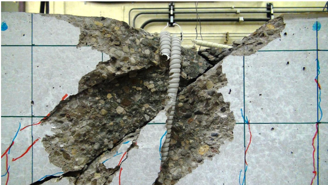
Figure E.93: BM16-220 Photo of Exposed Stirrup and Failure Plane after Loading from Reverse
