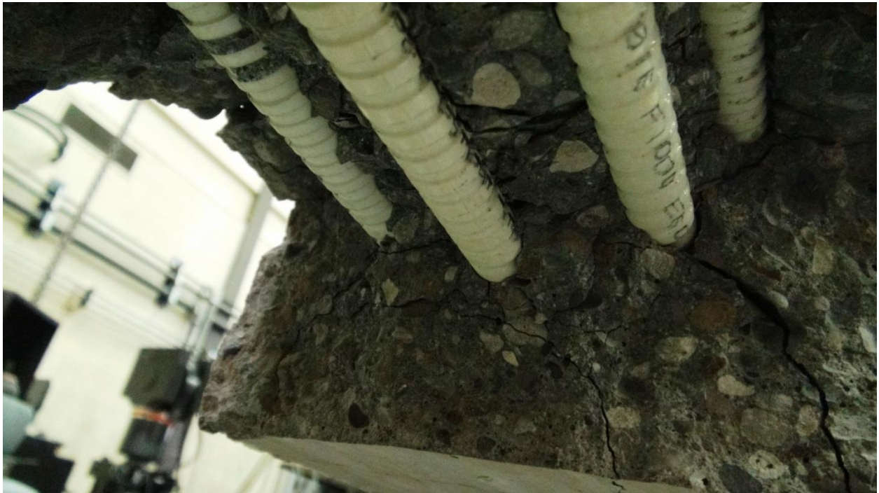
Figure E.227: BM16-s230 Photo of Exposed Longitudinal Bars and Tensile Splitting Cracks
