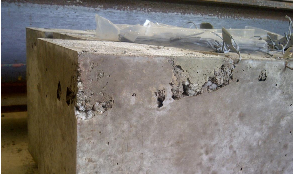
Figure 3.7: Typical Extent of Honeycombing
