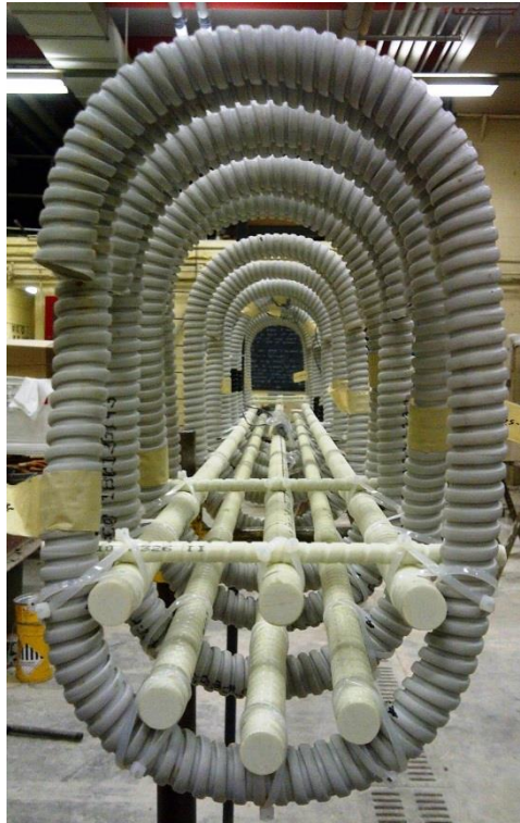
Figure E.223: BM16-s230 Rebar Cage Cross-Section Photo Top framing bar not pictured.
