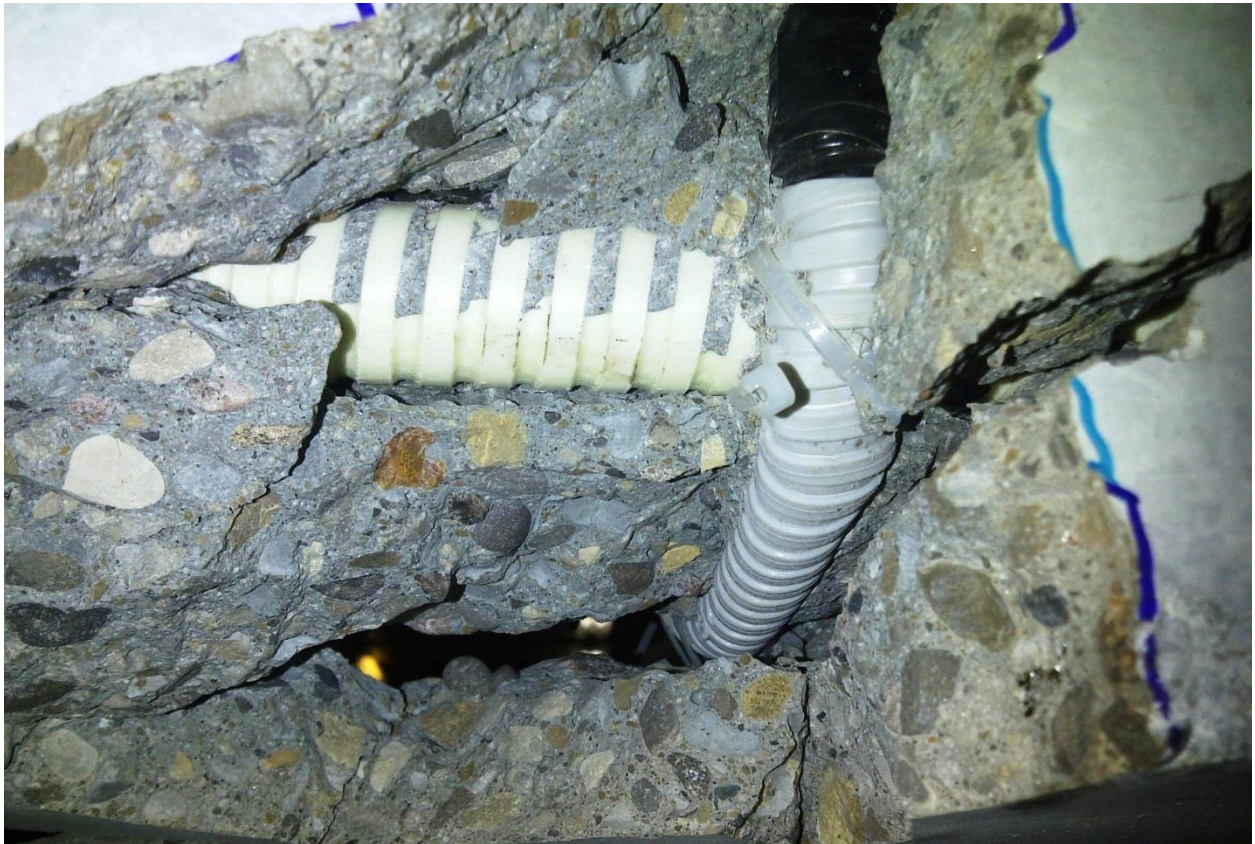
Figure E.115: BM25-220 Photo of Exposed Stirrup after Loading 2
