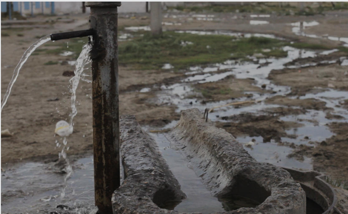
FIG. 14 Free-flowing water pumps/standpipes providing drinking water are found throughout Aral'sk. Water is pumped from one of four reservoirs in Aral'sk, which are supplied by the Aral-Sarybulak Water Pipeline, originating near Baikonur, Kazakhstan. The water network was built in 1963, and has been repaired with funding from the International Fund for Saving the Aral Sea (IFAS) in 2000-2002.
