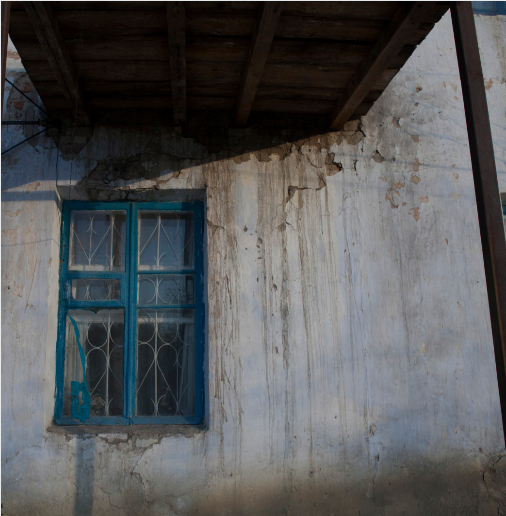
FIG. 28 The plaster on this two-storey colonial apartment shows water stains and efflorescences.
