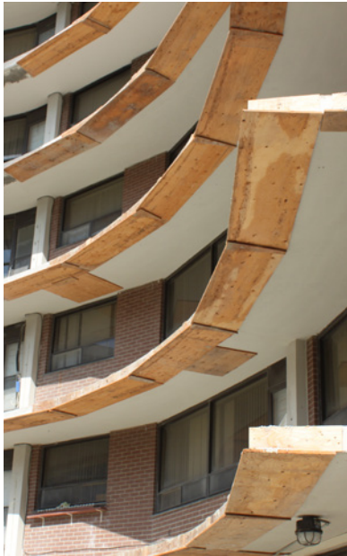
Figure 2-17 top left Cluster of Buildings in an Apartment Neighbourhood Undergoing Balcony Reconstruction: Eglinton West, Toronto
