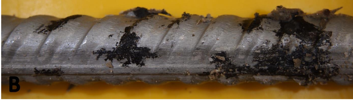
Figure 4-34: A: Corrosion products migration demonstrated on the concrete surface adjacent to the steel; B: rebar surface corrosion on Valbruna XM28
