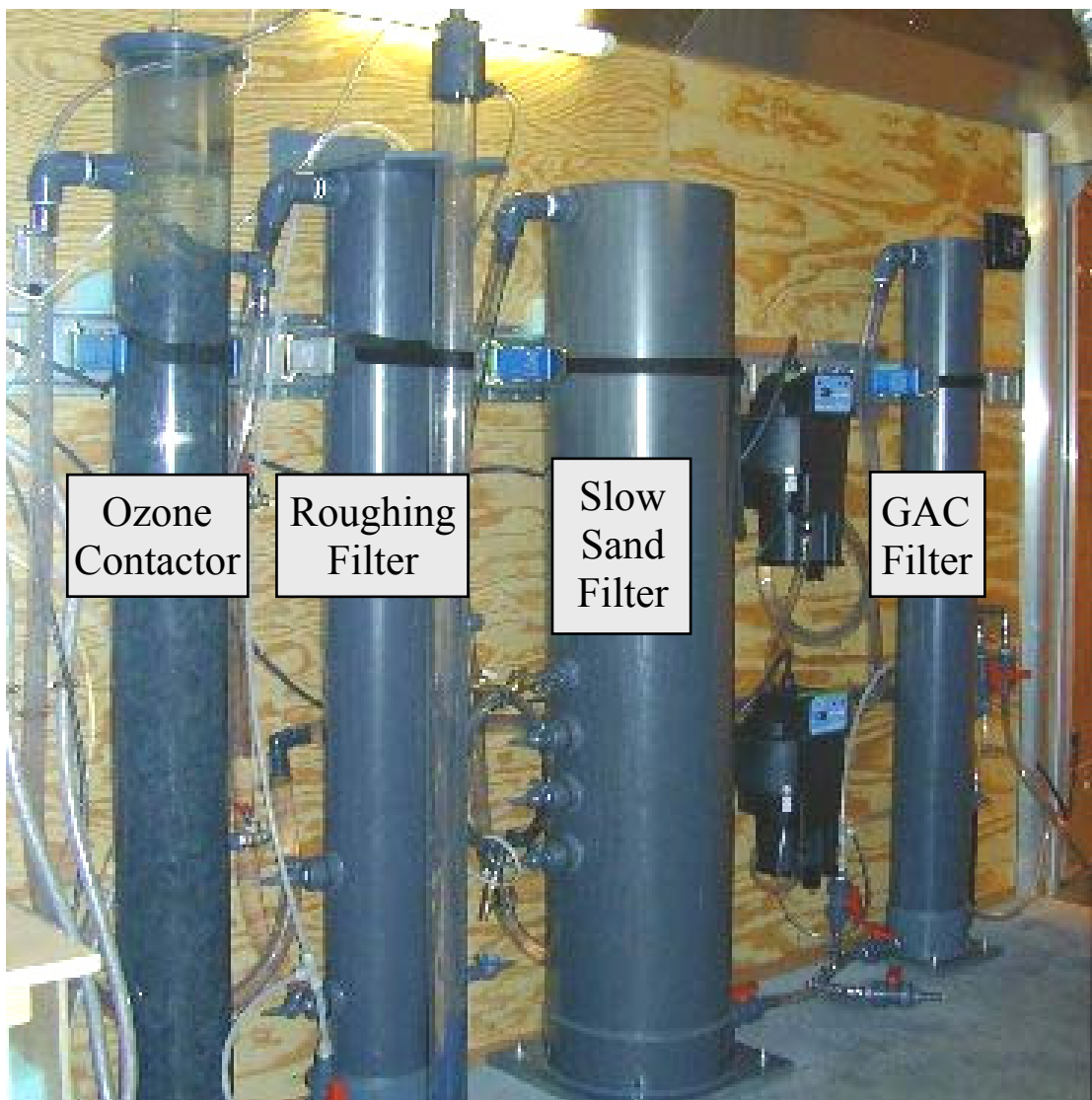
Figure 3.2: Pilot System 1 - Interior View
