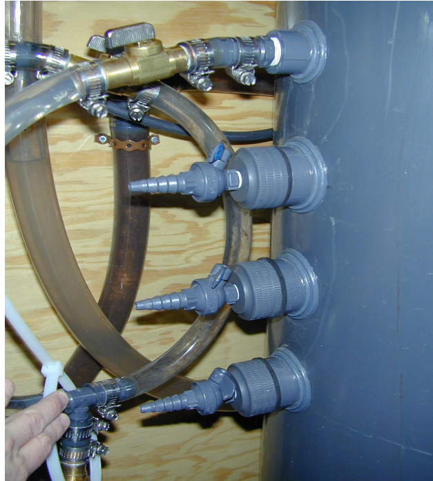
Figure 3.8: Typical Sampling Ports in Pilot System 1
