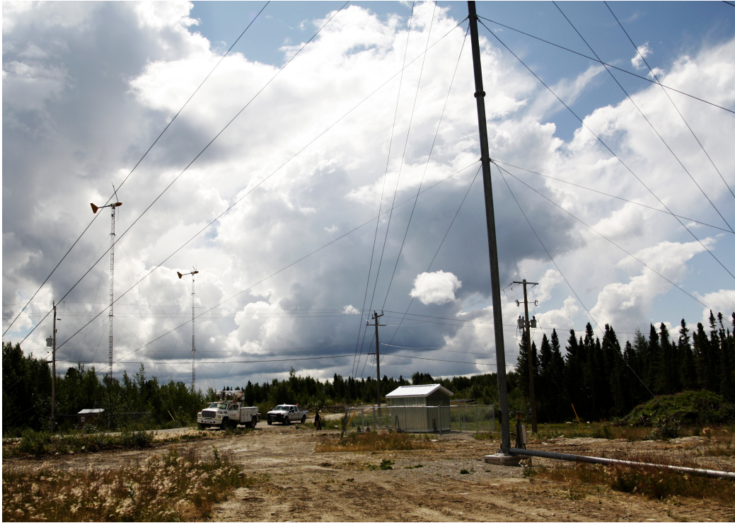
Figure 1.3: Small WTs with tilt-up towers installed at KLFN, Ontario.
