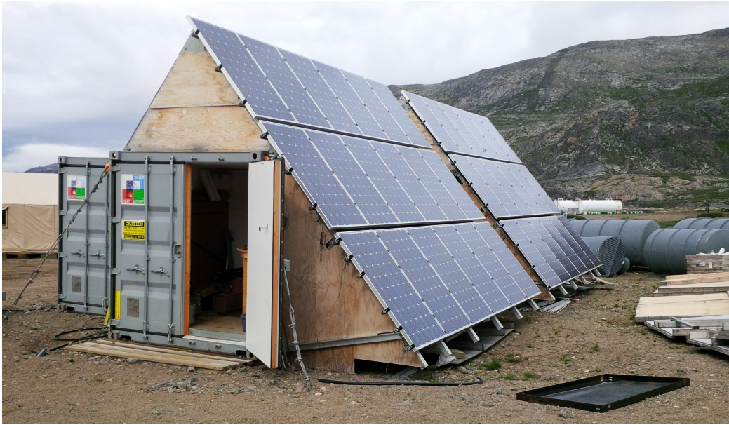
Figure 1.2: Solar PV system installed at the remote Torngat Mountains National Park base camp, Labrador (photo courtesy of Oliver Johnson).
