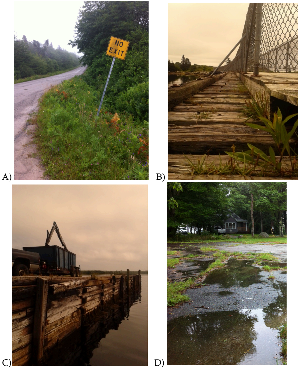
Figure 5.3: Photos describing the need for town upkeep. A) Dirt road with lots of potholes (Youth Participant 2). B) Trestle bridge in Lockeport missing some planks (Youth Participant 4). C) Allendale wharf missing planks and ladders (Youth Participant 4). D) Vacant lot in Shelburne (Youth Participant 3).
