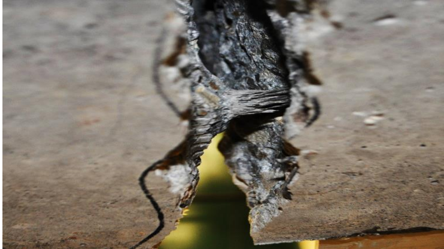
Figure 6- 3 Sand coating sheared off the basalt bars
