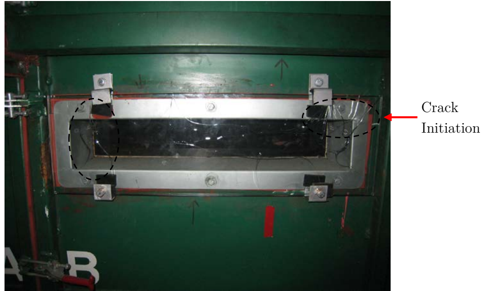
Figure 4.7: Locations of window crack initiation
