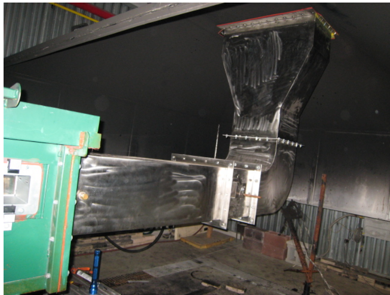
Figure A.3: Exhaust duct transition piece aligned and installed between the two openings
