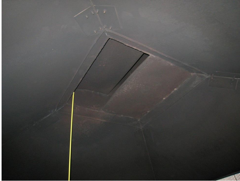
Figure A.1: Exhaust entrance opening underneath the fume hood
