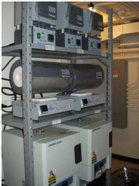
Figure 10: Programmable furnaces (bottom) and manual furnaces (top)
