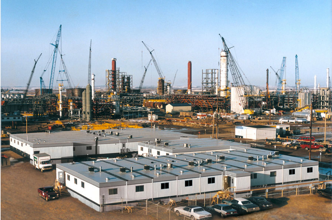
Figure 14: Industrial Accommodation by Modspace at Husky Refinery
