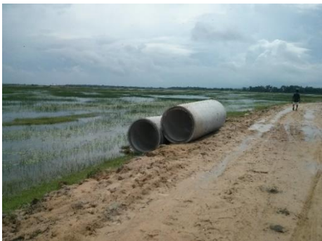
Figure 4.4: Concrete tunnels used to connect the lagoon; Source: Picture taken during the field research
