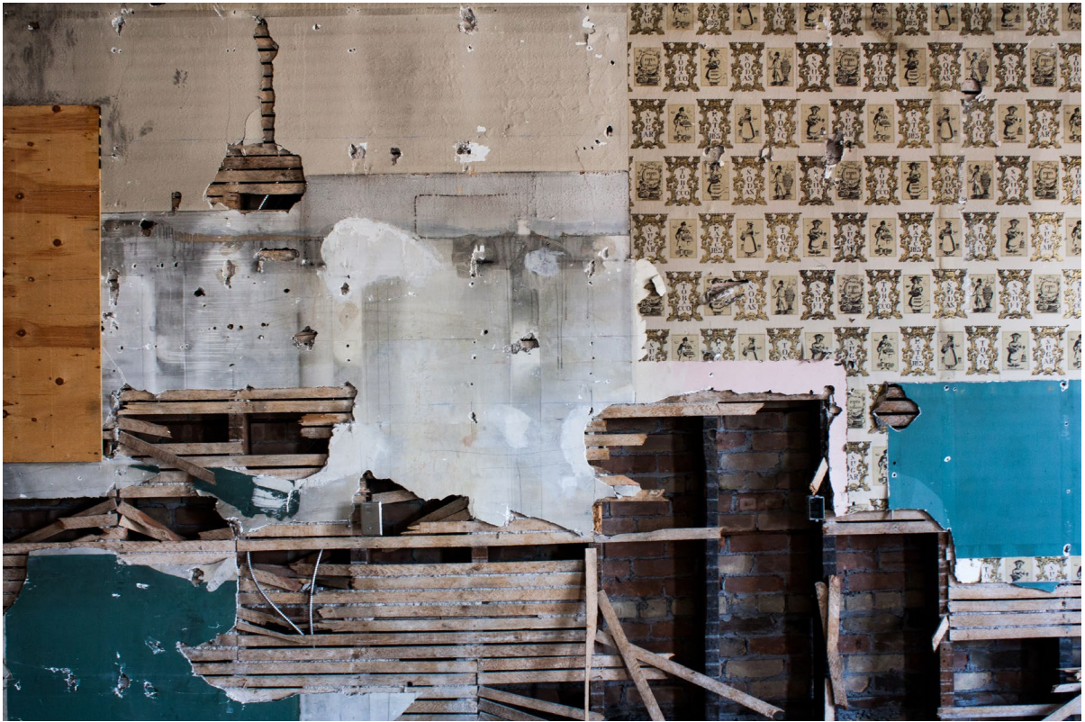
Plate 14: Layers of the building's history exposed on the second floor at 60 Main Street. [2015-06-26]
