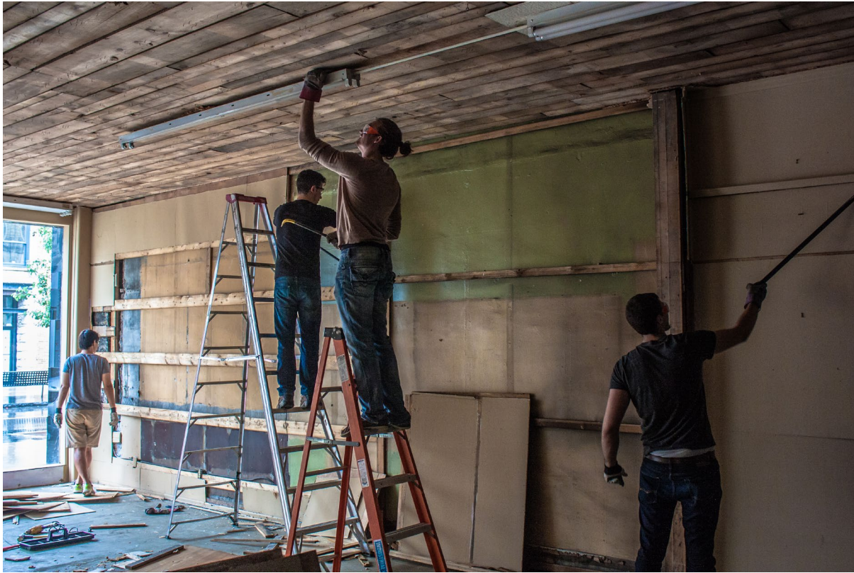
Plate 78: Ripping off the plywood wall covering and removing ceiling tiles under the light fixtures. [2015-06-27]
