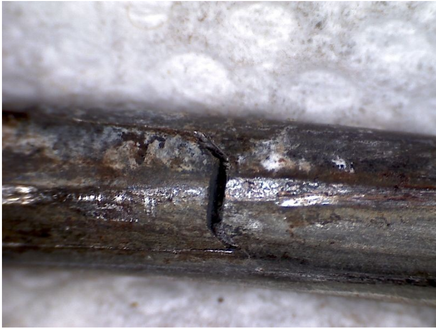
Figure 5-8 – Close-up of inter-wire fretting damage on an external wire of a 7-wire prestressing strand as extracted from the beam after failure
