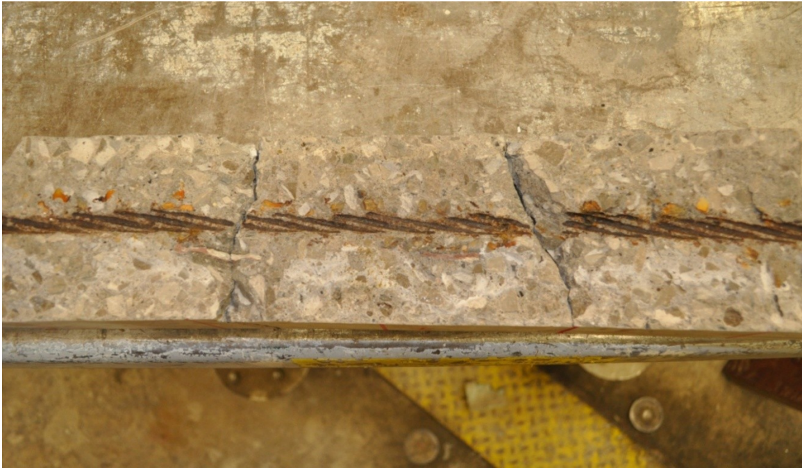
Figure 4-22 – Concrete strand interface below the strand
