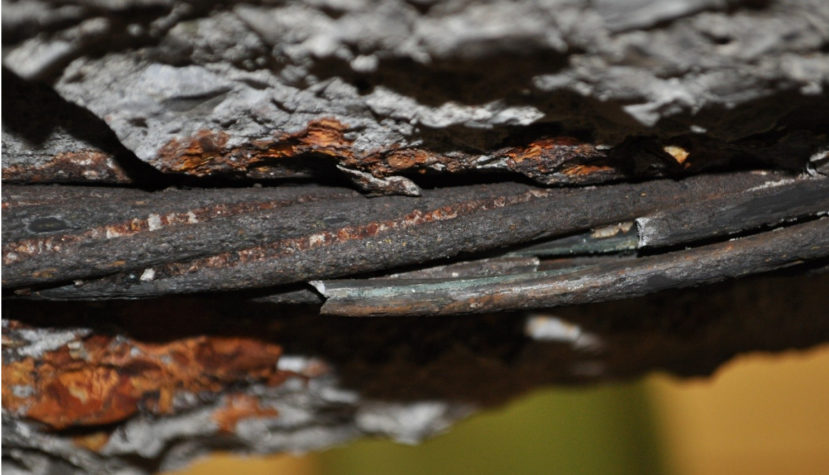
Figure 4-25 – Wires rupture at adjacent locations in a corroded beam
