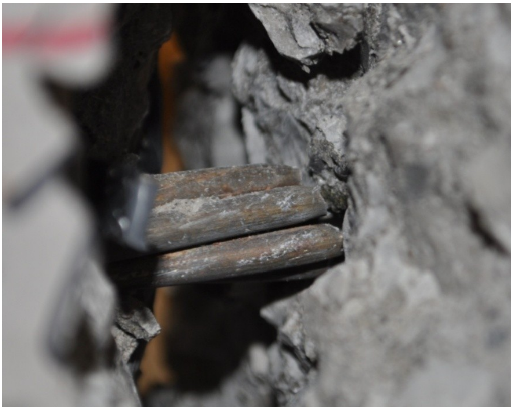
Figure 4-24 – Multi-wire rupture at the same location for the uncorroded beam
