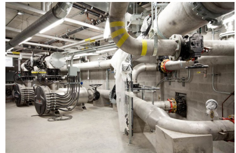
2.20 UV facility of the project located underground to filter the water.
