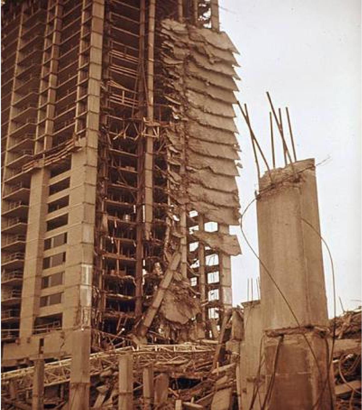
Figure 1.4: Skyline Plaza collapse, Fairfax County, VA, USA, 1973. (Courtesy of NIST)
