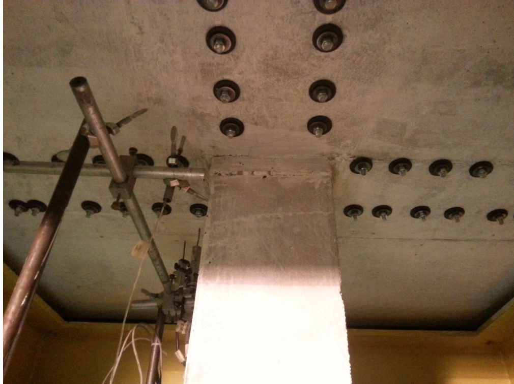
(a) Cracks at 1% drift
