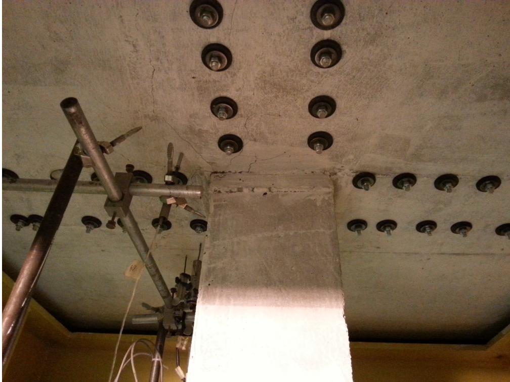
(a) Cracks at 3% drift
