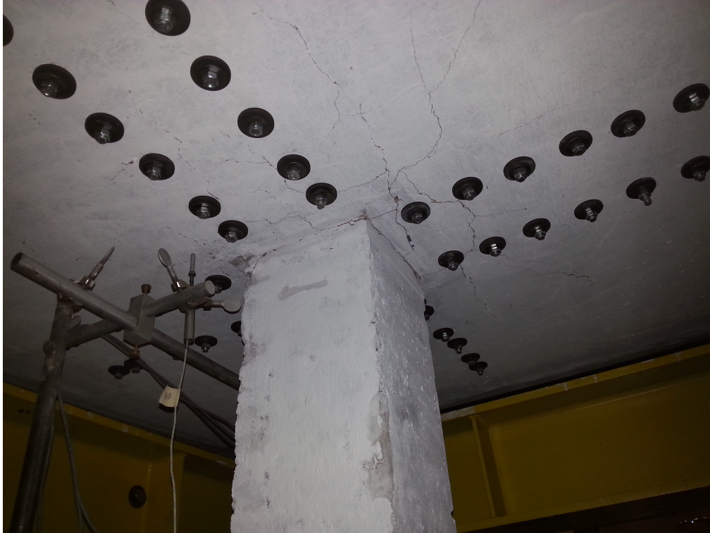
(a) Cracks at 3% drift
