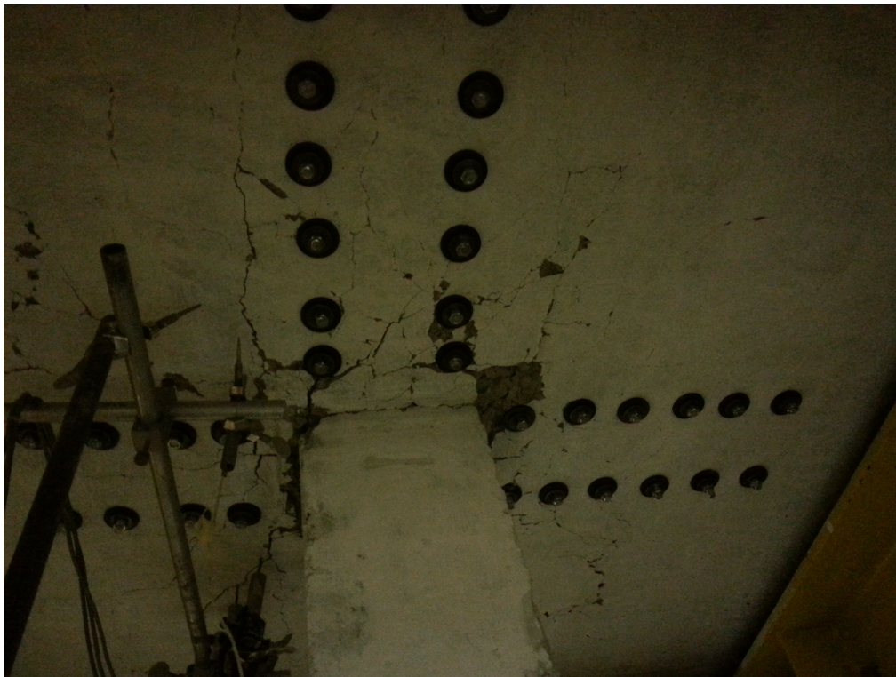
(b) Cracks at failure
