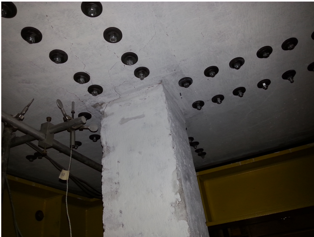
(b) Cracks at 2% drift
