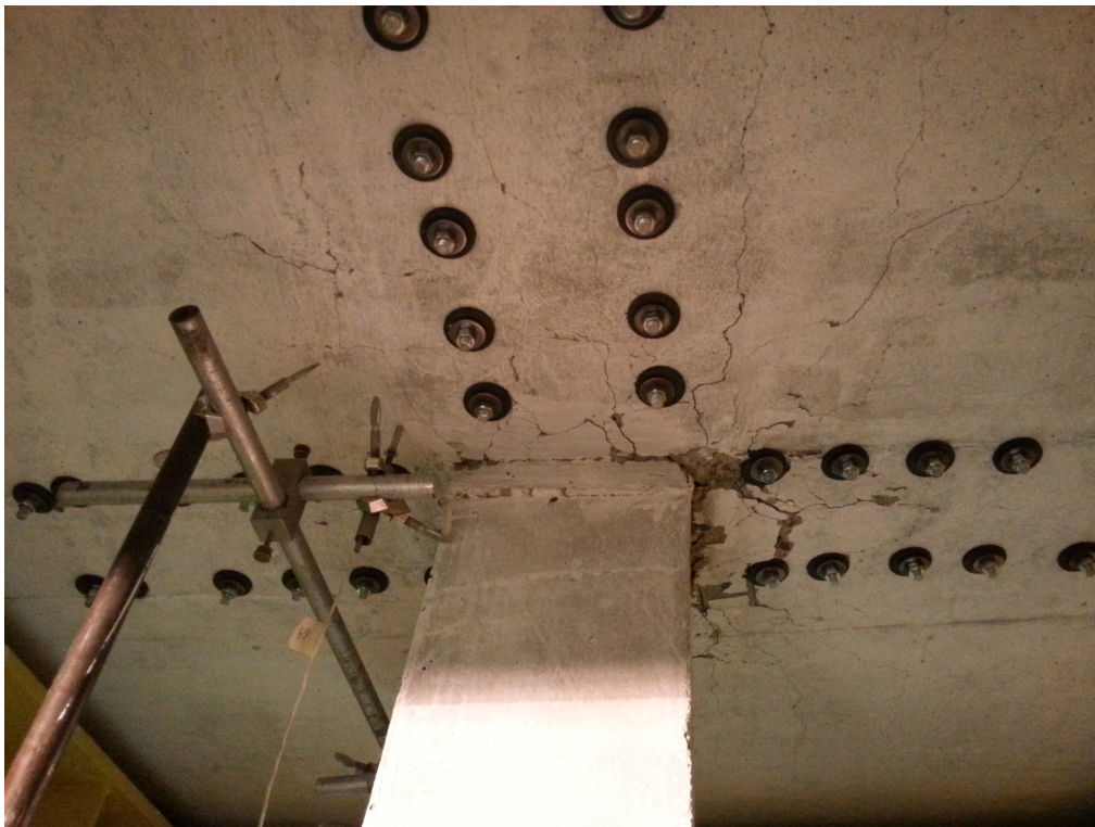
(b) Cracks at failure
